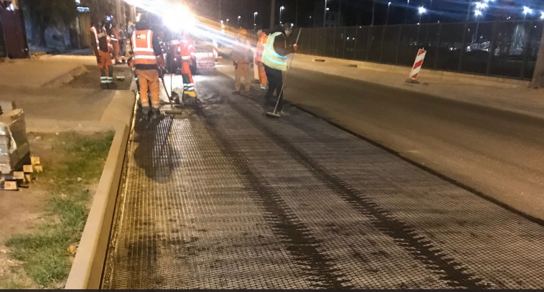
Tensor AX5-GN geocomposite was laid on the freshly sprayed bond coat layer of bitumen emulsion.
